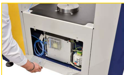
Opening door for better access and easy maintenance
